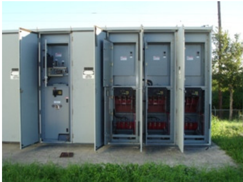
MCC-03 Sections 12, 13, & 14 for Future 350HP Pumps
